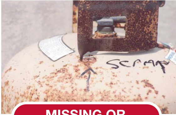
MISSING OR DAMAGED COLLARS
