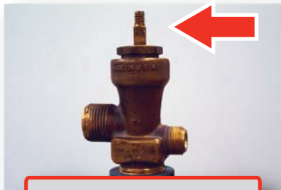
MISSING HAND WHEEL
